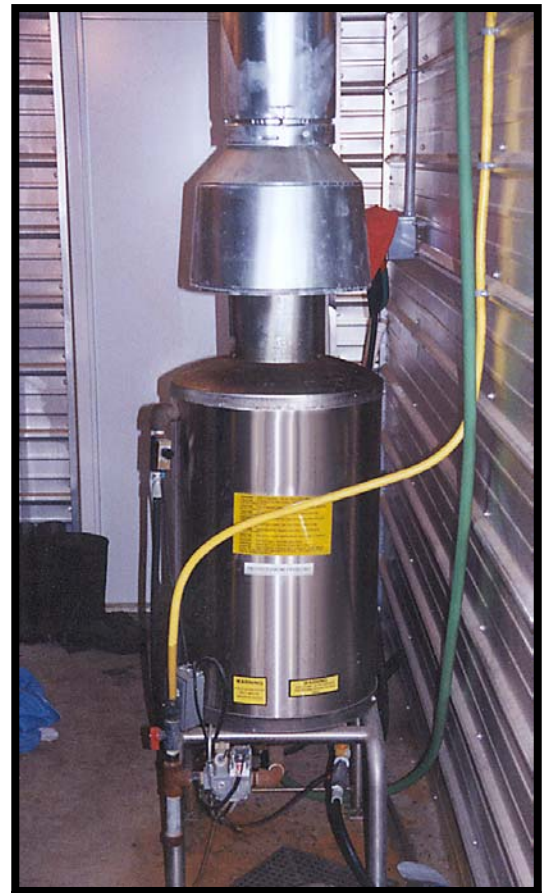
Photo 1 – Side view of LP fired heater unit.
